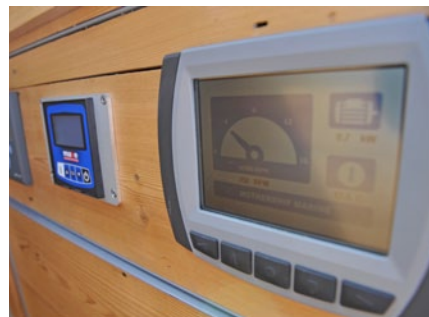
High-tech monitors on board
